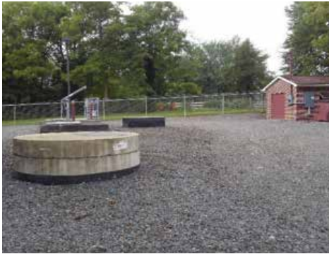
Pump Station #4 at work
