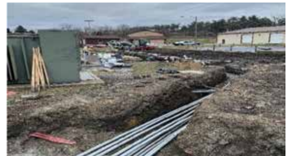
Conduit bank for new air blower system
