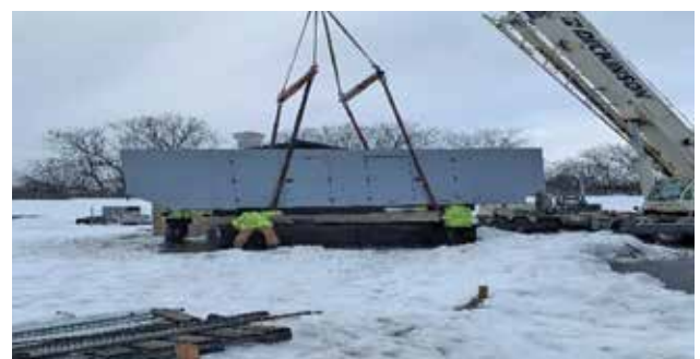
New 500 KW plant generator
