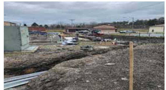
Conduit bank for generator transfer switch
