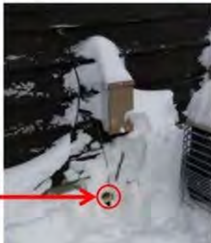
Nearly blocked vent pipe
